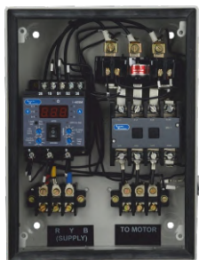
Interior View of MD Starter+ DOL Starter
