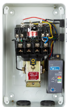
Interior View of MK1.i
