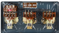
Interior View of MK2 SASD
